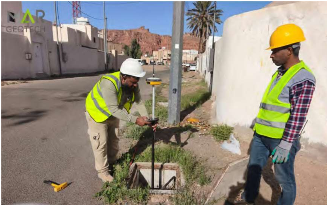
Manhole Inverted Level
